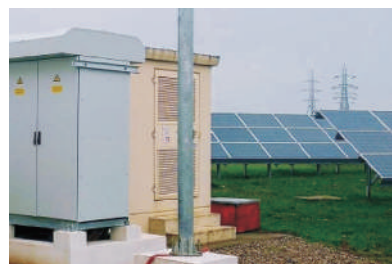
Energy Storage Cabinet
